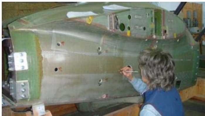
One repair procedure on the right fuselage and over 80 visible open holes in the one wing and mid fuselage.
