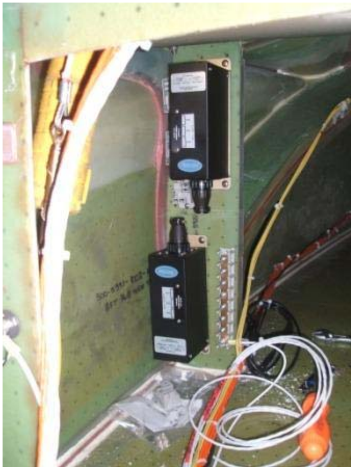
The sensors drive the dual computers in the aft hull compartment.
